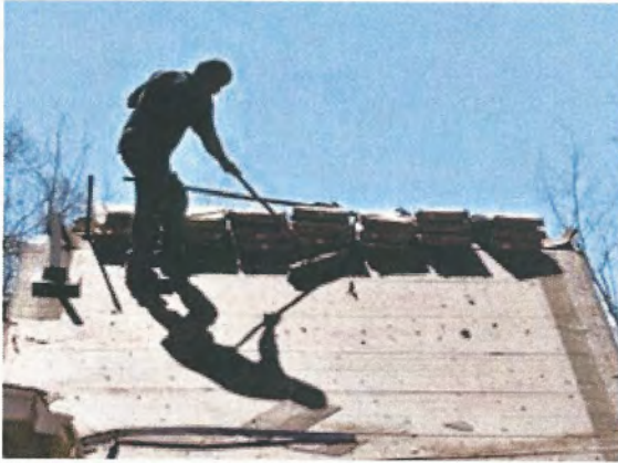
Workers put on a new roof on a house on Lucy Grant's home on Hanson Street.
